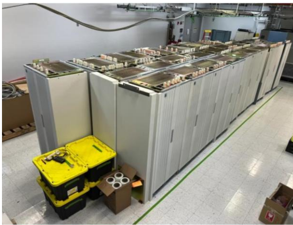
Switch components are ready to be transported
