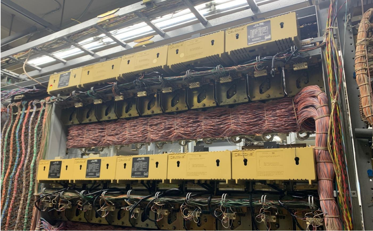
The Teltone CONVERT-A-PAK equipment at THG's museum
