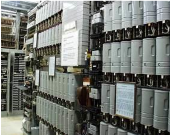
Banks of automatic (step-by-step) switches
