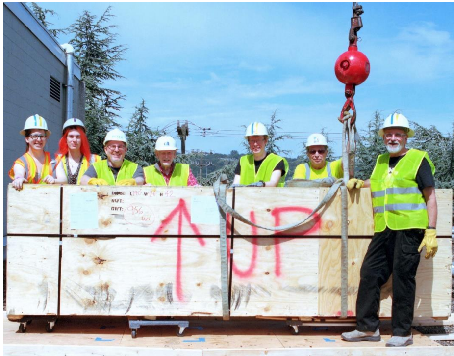
Seattle volunteers with the first of the two frames once lifted on to the museum roof. (Left to right: Sarah Autumn, Astrid Smith, Peter Amstein, Les Anderson, Colin Slater, Dave (Western Crane), Eric Rhinelander) Photo by David Dintenfass
