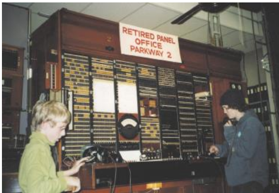
Andrew checks out a panel switch.
