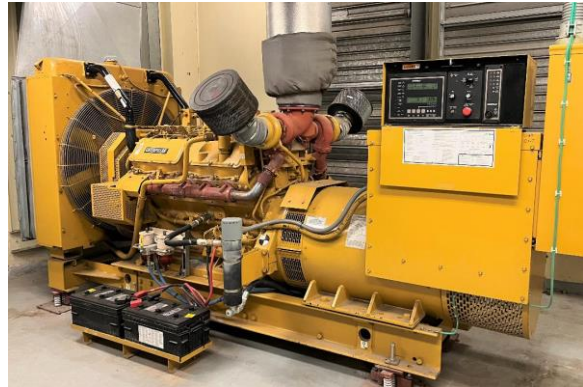
Contemporary batteries and generator
