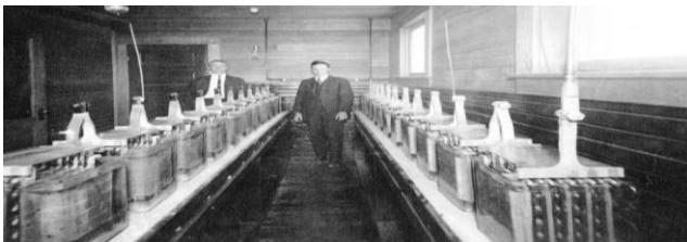
1920's Central Office battery room and generator
